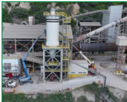
As part of its ongoing expansion project, scheduled for completion in the first half of 2025, Caribbean Cement Company Limited has installed a 160-tonne capacity surge bin along with solid fuel equipment.
